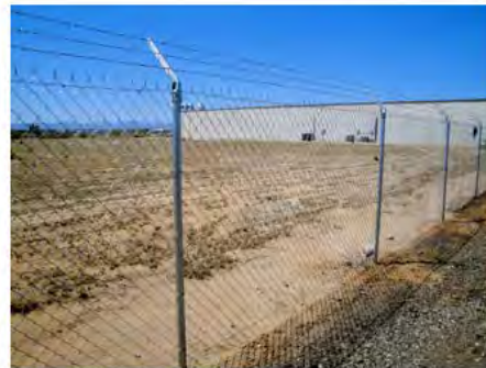
Galvanized Chain Link W/ Barbed Wire (Substation Only)
