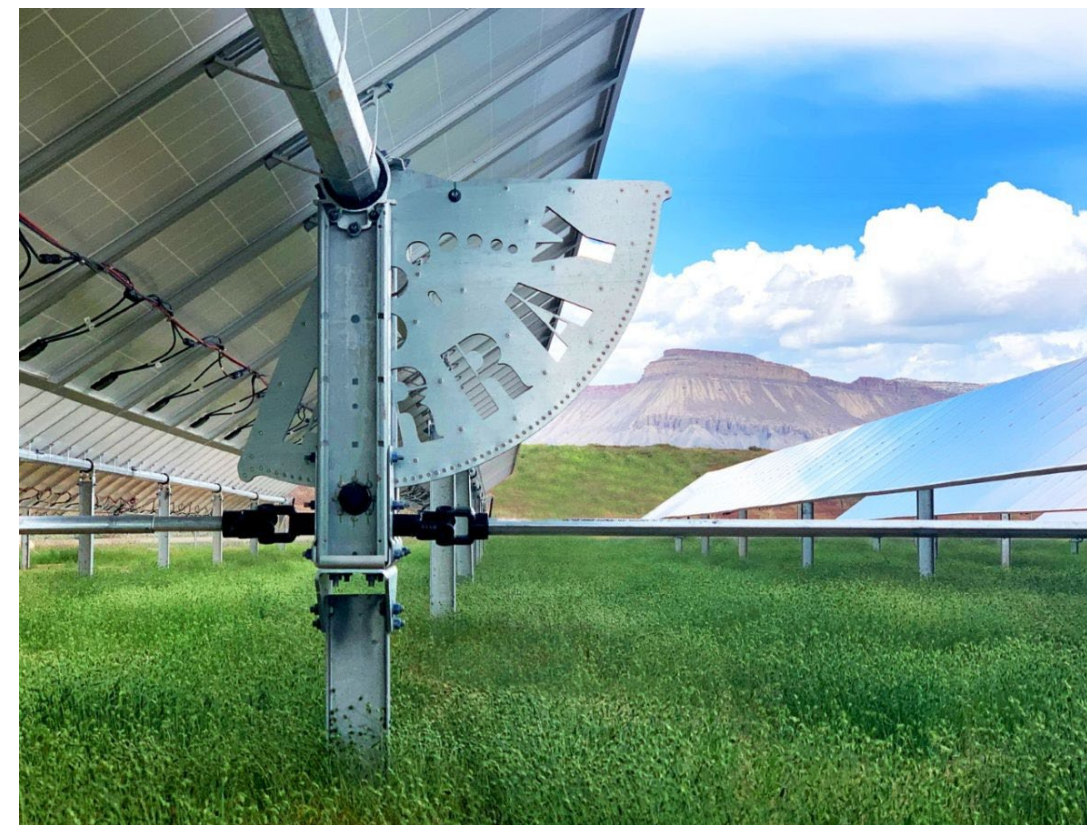
Racking mounted on piles
