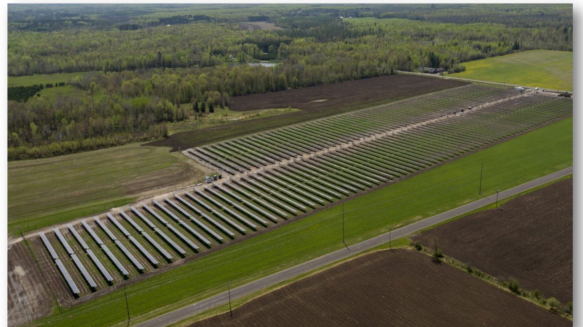
One section of array at EDFR's Project in Flambeau, WI
