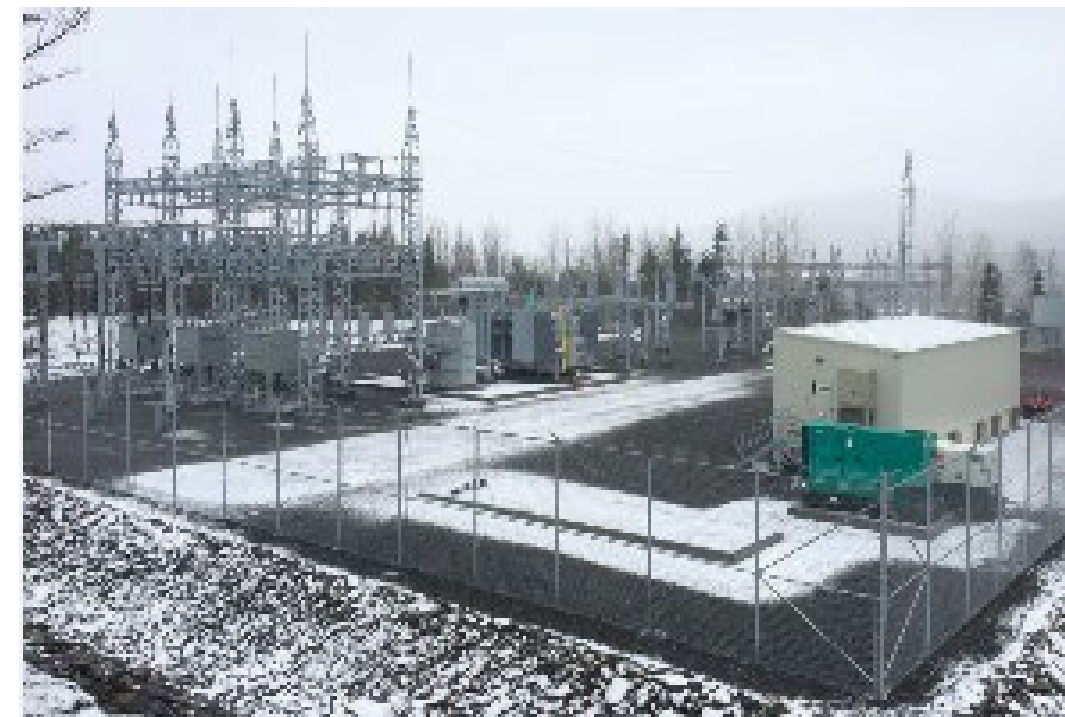
Project substation (grid tie)
