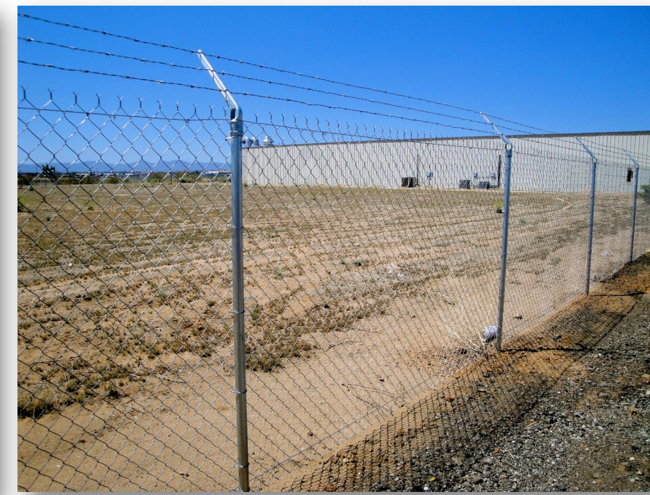
Galvanized Chain Link W/ Barbed Wire (Substation Only)
