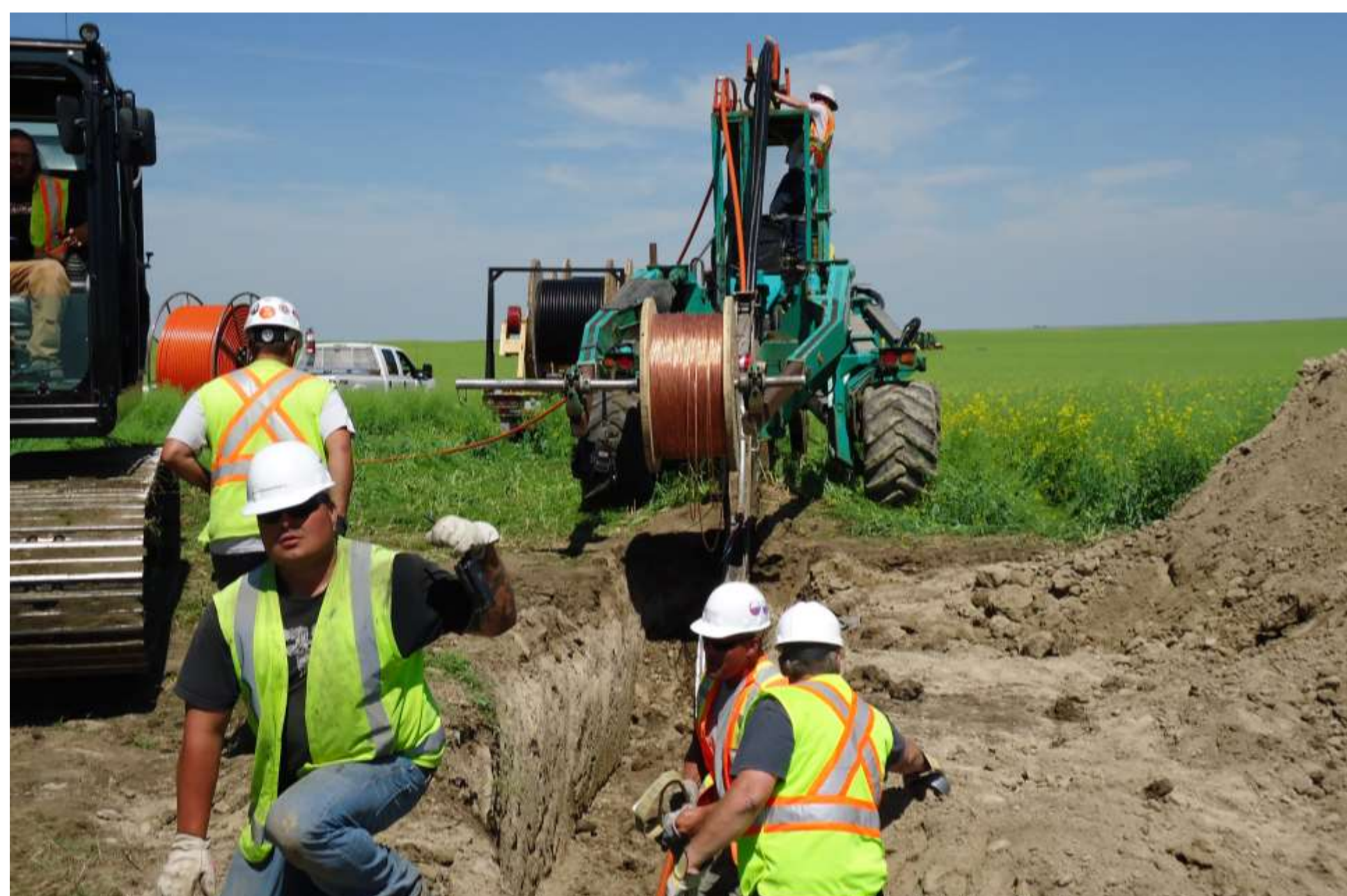
Buried collection system
