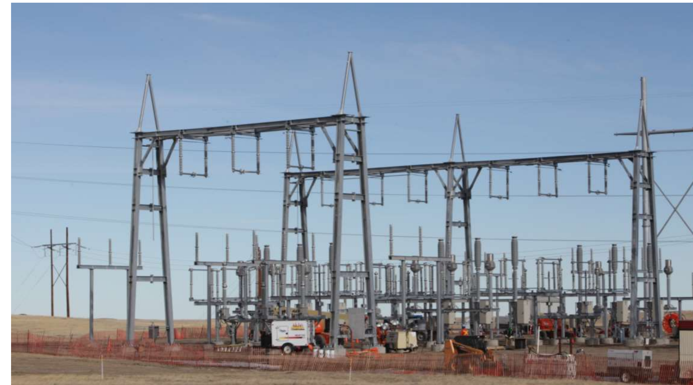
Substation connecting a project to a transmission line
